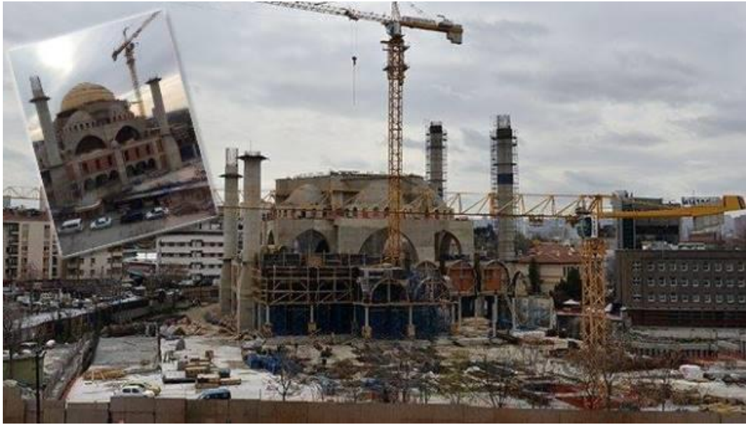
Figure 4.16. The construction of Melike Hatun Mosque and İller Bankası building next to it before its demolition. (Source: http://www.mimdap.org/?p=194061 )
